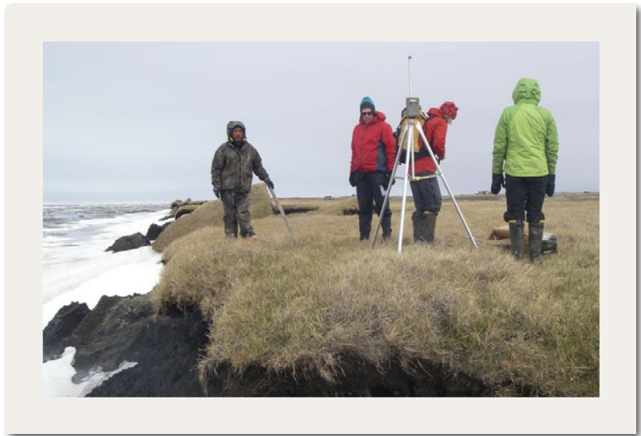
NOPP researchers install a time-lapse camera to monitor coastal erosion in the Arctic. Photo credit: R. Anderson
