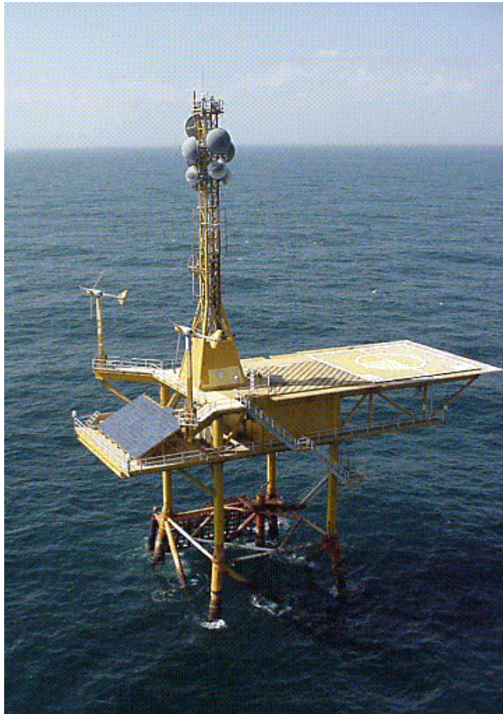
[Figure 1. The M2R6 platform. This “master” platform is located in 33 m water depth about 60 km offshore. Power on the three master platforms is generated by photovoltaic panels, wind generators and a diesel backup generator. A high-bandwidth microwave network is used for communications between master platforms and shore. Helicopter transportation of personnel is used for most servicing operations.]
